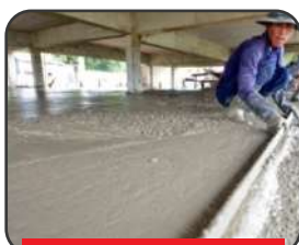
Mengurangi early-age cracking
